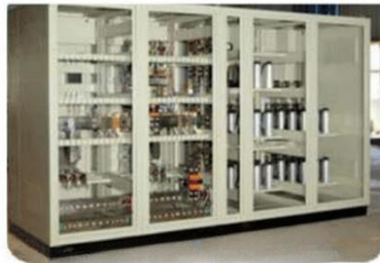
INSIDE VIEW MSB-MAIN ACB 4000A
